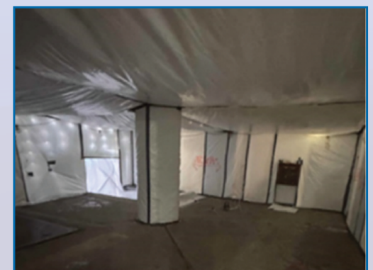
Isolated Clean Area of the 1st Floor
